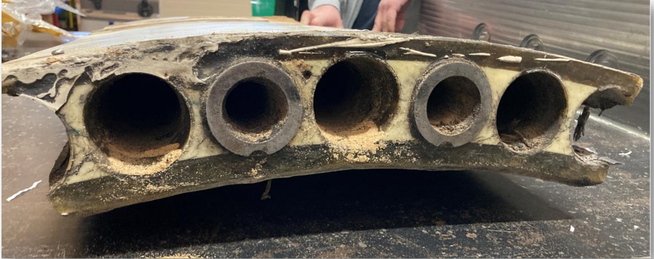
Root which is affected in the bushing area
